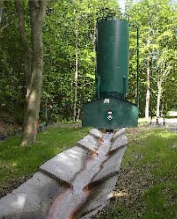
Essex Doser, Photo by Monday Creek Restoration Project
